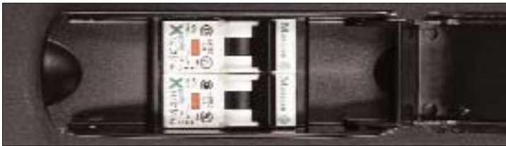
UL 489 hydraulic-magnetic circuit breaker on 30 Amp PDU.
