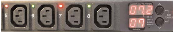
Rear of 1U PDU showing current draw for outlet #7. Red LEDs show outlets that are switched on. Green LEDs show outlets that are switched off.
